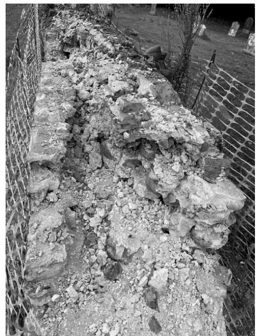
Cavities inside the wall
