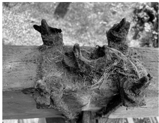
The existing rusted headstock which was just about holding the bell in place
