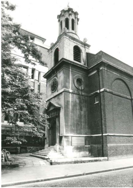
Fig 1 The west end of the church showing broken and dirty stonework.
