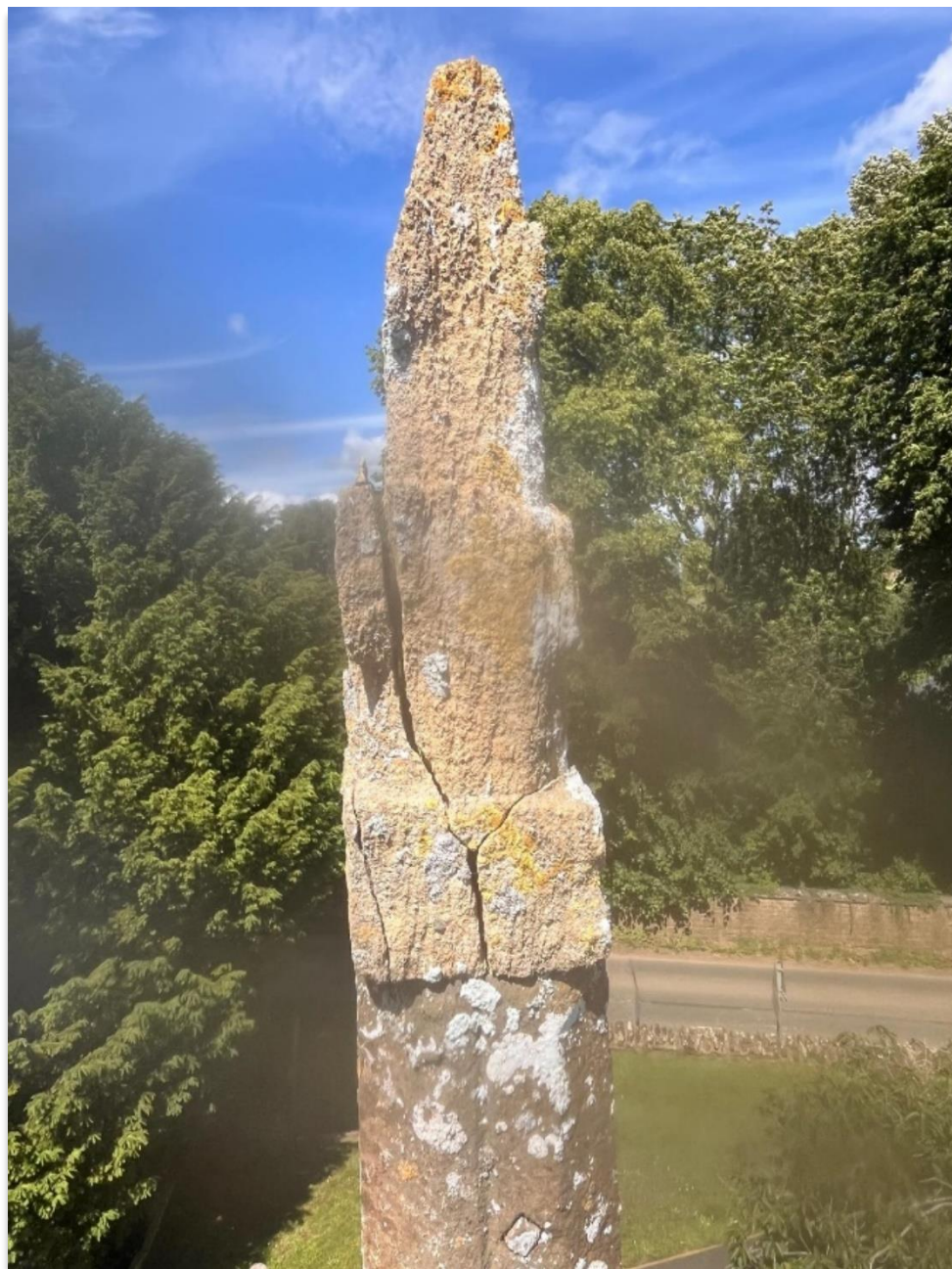
A split pinnacle on the roof of St. Nicholas Churches due for repair. N.B. The area below has been roped off.
