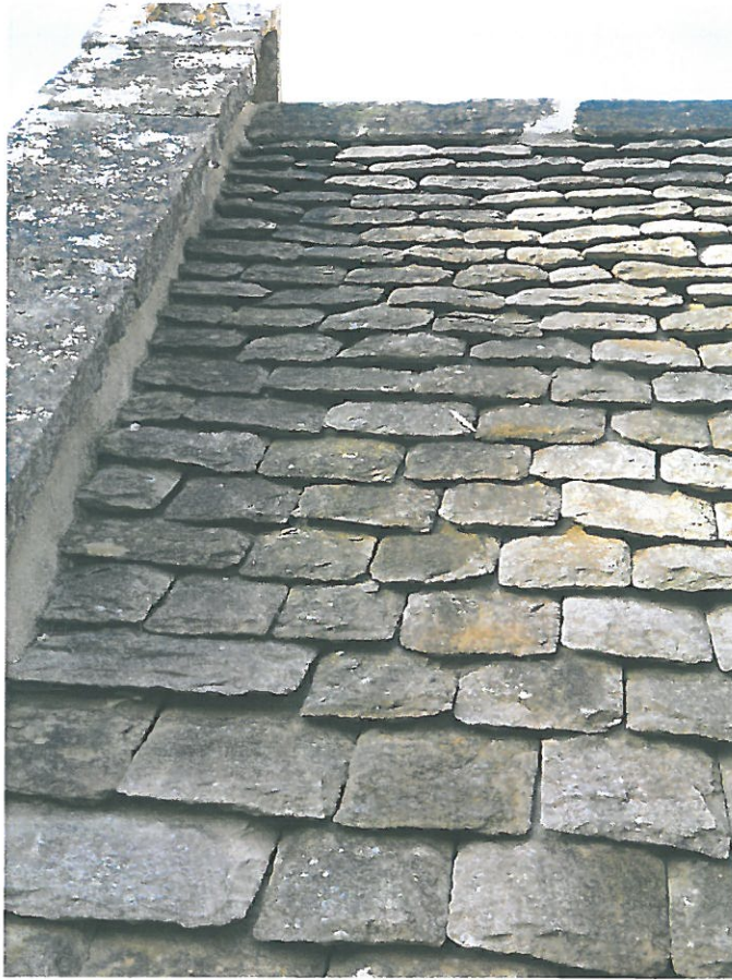
Detail showing delaminated tile to south porch.
