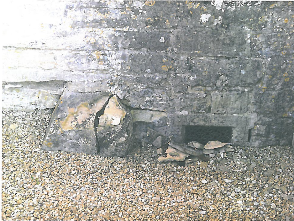
Fractured plinth block to tower.
