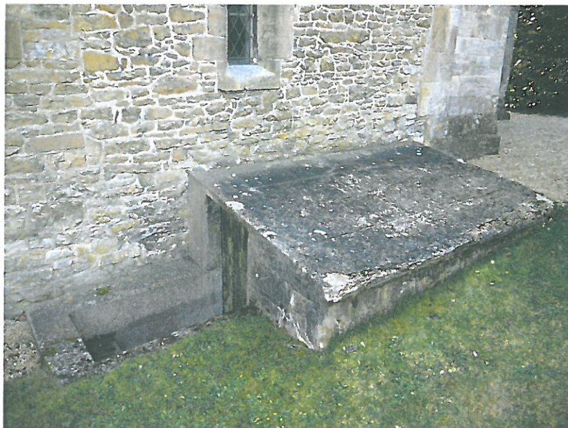
Spalled capping to old boiler room.
