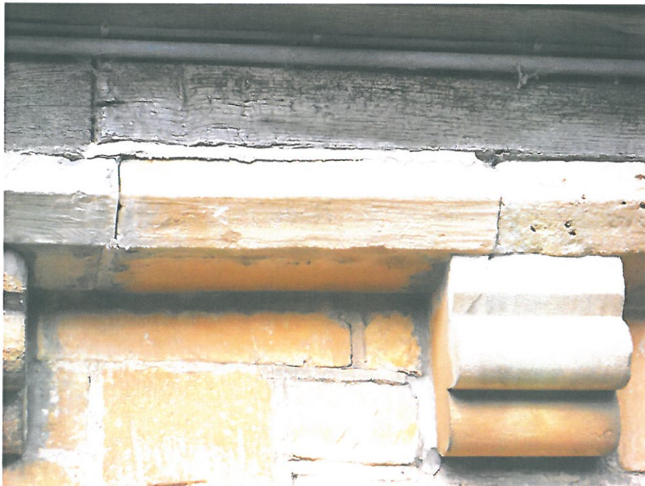
Detail of dislodged eaves stone and fractured corbel.
