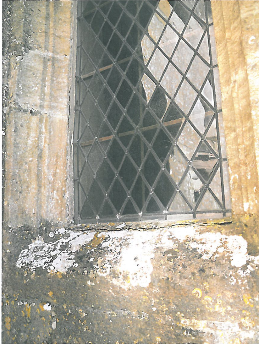
Detail showing defective pointing to west window of nave.
