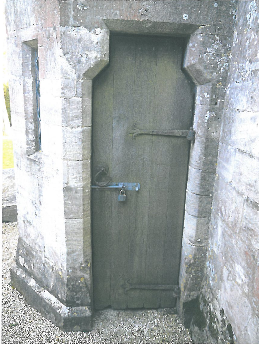
Poor decorative condition of metal work to door to tower.
