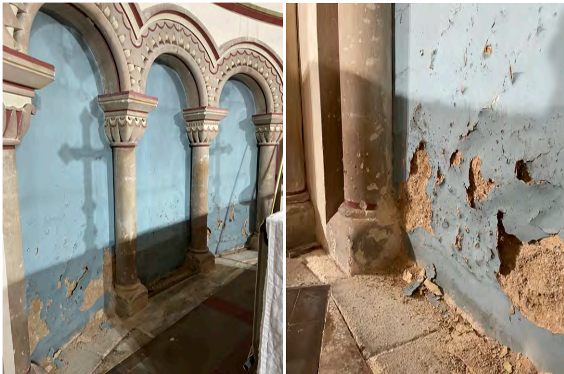
Overview of the blue painted panels, left, and right, detail of the condition of the first of these panels
