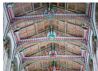
The superb internal roof following recent renovation and repainting at St. Cuthbert's Church.
